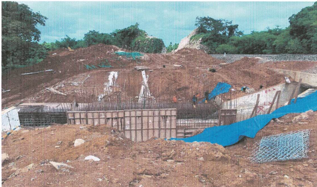
Monitoring pekerjaan CT 501, pekerjaan pembesian box culver , wing wall box culvert , stok sub ballas
